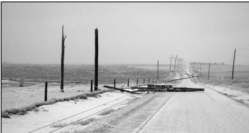
A typical scene of poles and power lines down after the massive winter ice storm.
