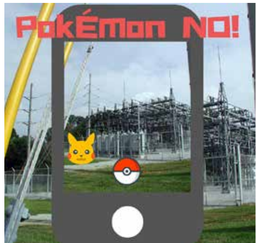
Be aware of your surroundings as you #CatchEmAll. Steer clear of electrical equipment, such as substations, power plants and pad mount transformers.
